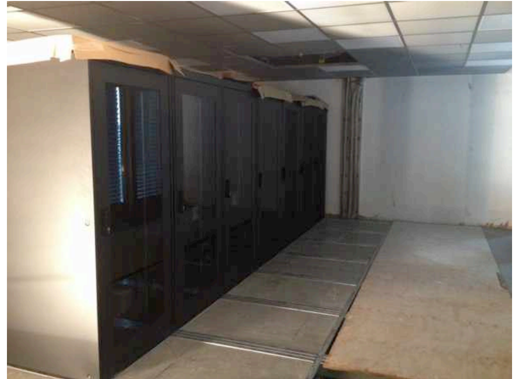
Installation neue Racks
